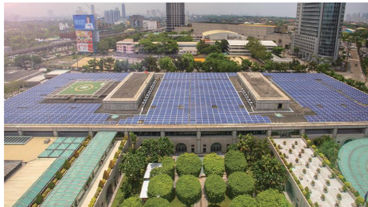
Asian Development Bank Rooftop Project Philippines System Capacity: 571 KW
