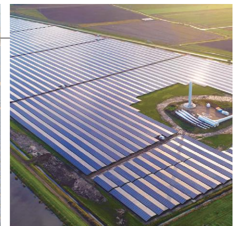
Solarpark Duurkenakker Netherlands System Capacity: 64 MW
