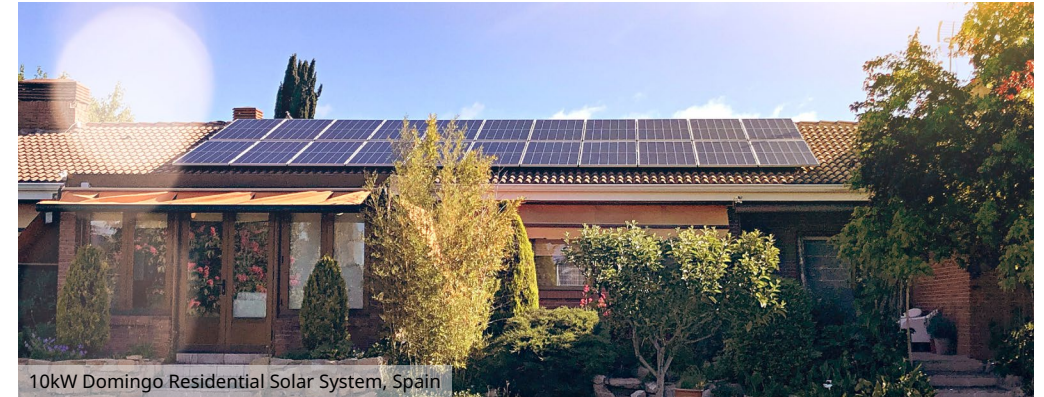
10kW Domingo Residential Solar System, Spain
