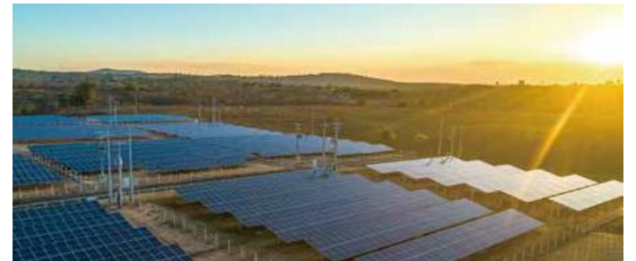
Setta PV Power Station Project
