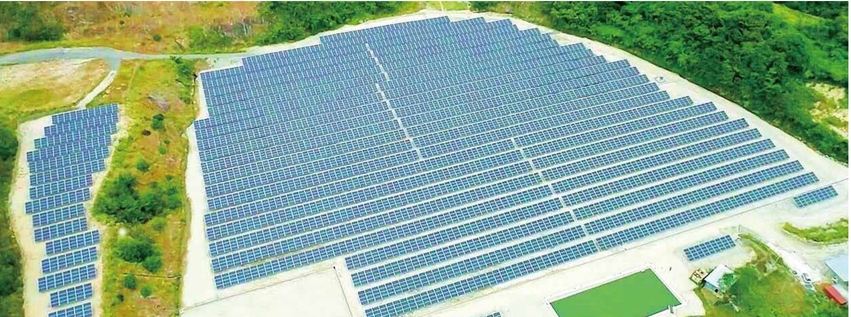
Japan 3.24 MW Power Plant Project Kanzaki Solar
