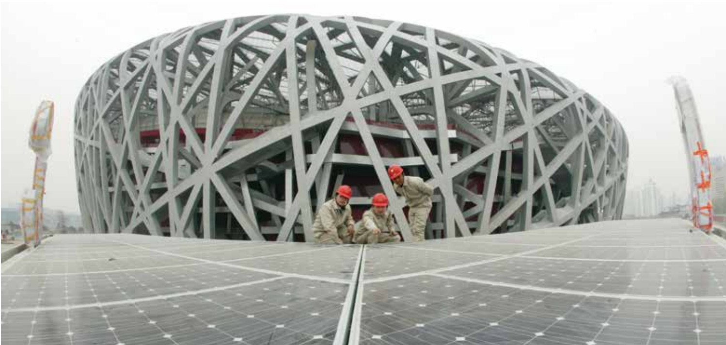
Beijing Bird's Nest Stadium BIPV Project
